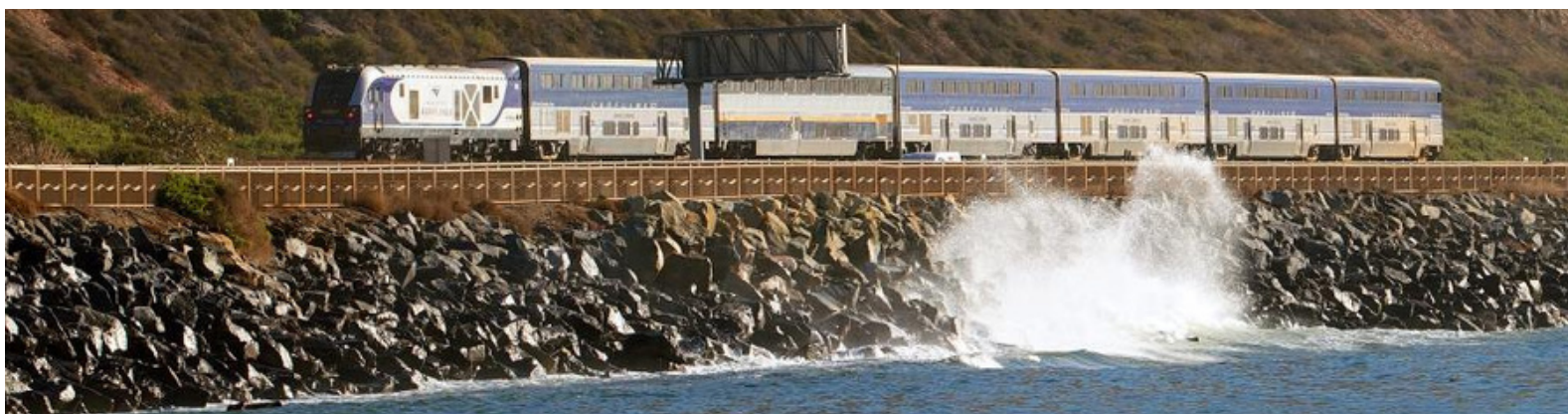
Coastal erosion threatens vital transportation infrastructure, such as this road and railway in Santa Barbara County (CA King Tides Project).
